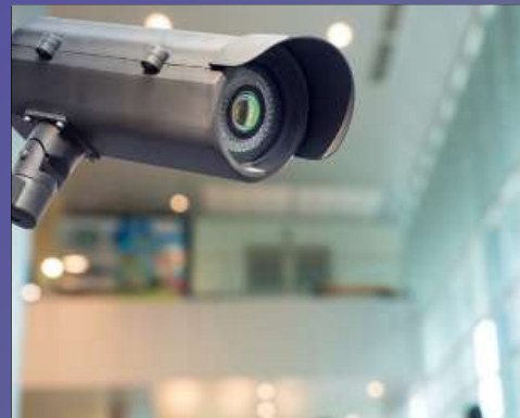
Security Equipment & Safety
